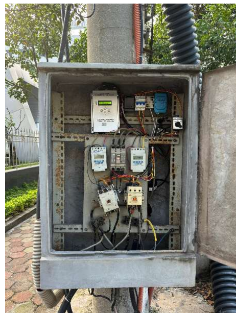
Figure 10. The device installed at Le Thai To 1 cabinet
